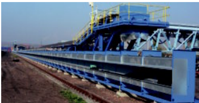
Longest igus® travel of 615 m with rol e-chain® and chainflex®-cables
