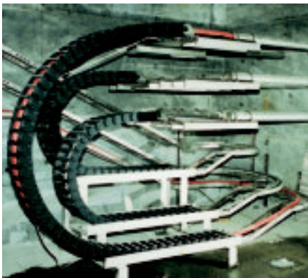
The igus® program offers up to 12 different bending radii from stock. Here, Series 50 used in the Storebaelt bridge project
