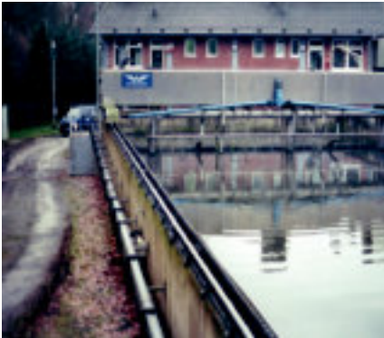
The scraper moves on the 38 m long final clarifier in round-the-clock operation. The energy supply is done via the lbt flizz® system
