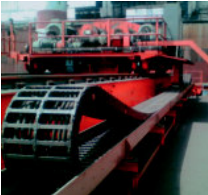
igus® rol e-chain® Serie 5050R in a steel plant in india with highly corrosive atmosphere - s = 22\text{ m} , v = 1\text{ m/s} , a = 1\text{ m/s}^2
