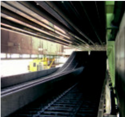
Assembled system in a ship unloading crane with igus® 5050RHD - Travel 106 m, Speed 4 m/s, Fill weight 25 kg/m
